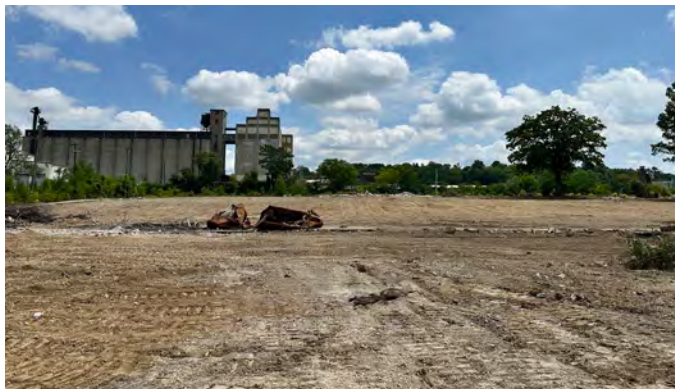
Remediation and demolition work is ongoing to reposition a former chemical plant site in Reading, Ohio for new investment and job creation.
